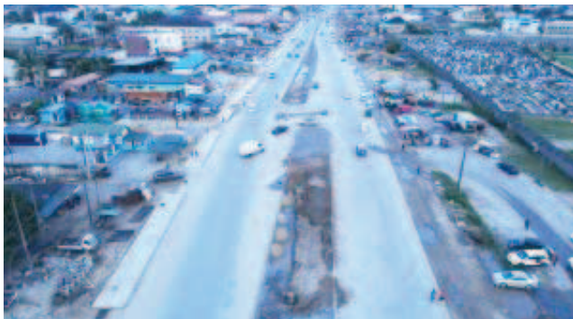
Deteriorated Eti-Osa-Lekki-Epe Expressway
