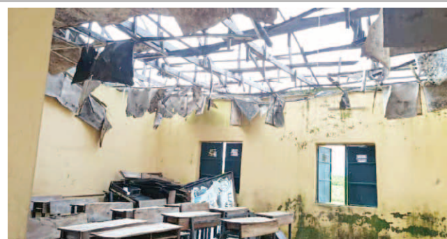
Leaking roofs and dilapidated infrastructure At LEA Primary School, Makanima, near Giri along Airport Road, Abuja
