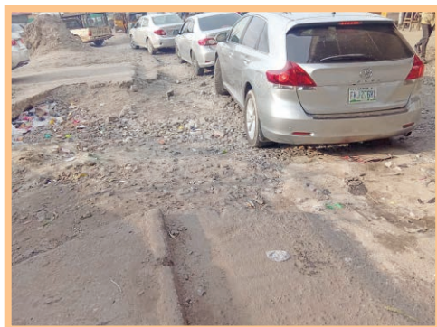
A big crater under the Jibowu Bridge at Mosalasi Bus Stop
