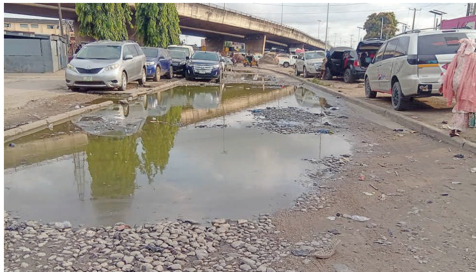
A waterlog section of the road that is impassable for motorists
