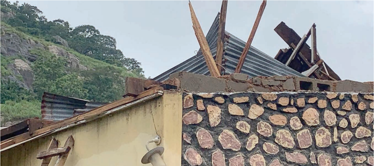
One of the buildings destroyed by the rainstorm in Isua Akoko, Ondo State.
